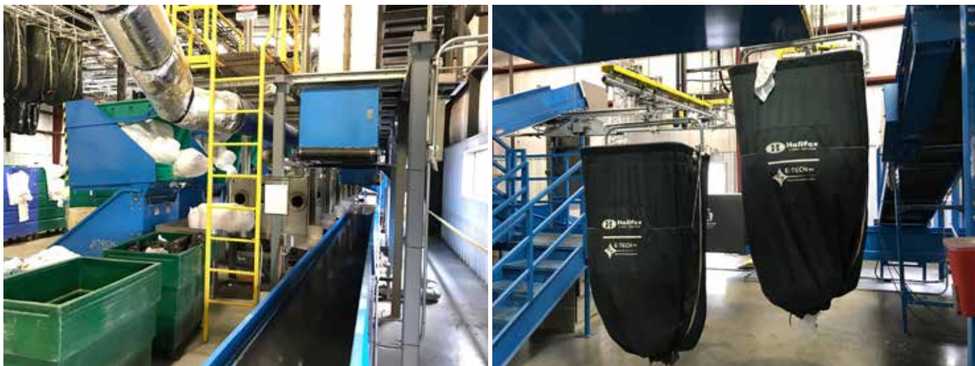
ABOVE: (l/r) Goods in the soil area are scanned in using RFID tracking software. Slings loaded with soiled goods await movement to the wash aisle for processing.
