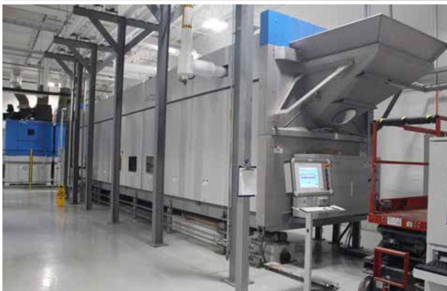
ABOVE: (from top) Employees feed sheets into a spreader/feeder in front of an ironer; another piece of ironing equipment; a view of the plant's tunnel washer.
