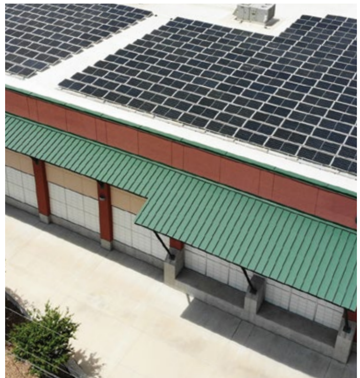
Solar panel installation at UniFirst-San Antonio, TX is a source of clean, sustainable energy.
