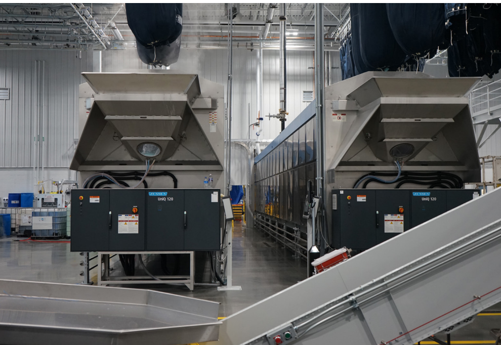
Above: Two tunnel washers at HandCraft Healthcare Linen & Uniform Specialists' new plant in Martinsburg, WV. Higher-pressure, "wide cake" tunnel presses have improved extraction, thus saving water and energy by reducing drying times.
